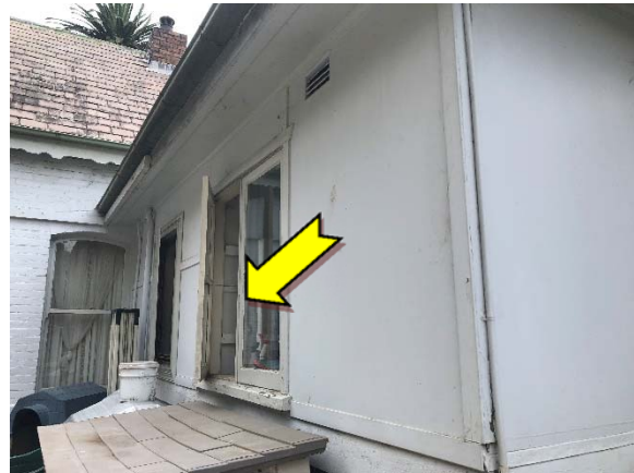
Photo 10. Exterior, windows and door frames – lead-containing beige upper paint systems.
