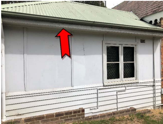
Photo 3. Exterior, rear extensions, throughout, eaves – suspected asbestos-containing fibre cement sheeting.
