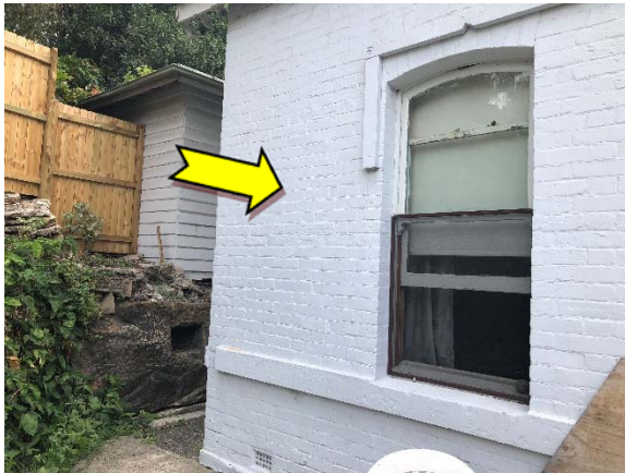
Photo 9. Exterior, throughout, walls and awnings – suspected lead-containing white upper paint systems.
