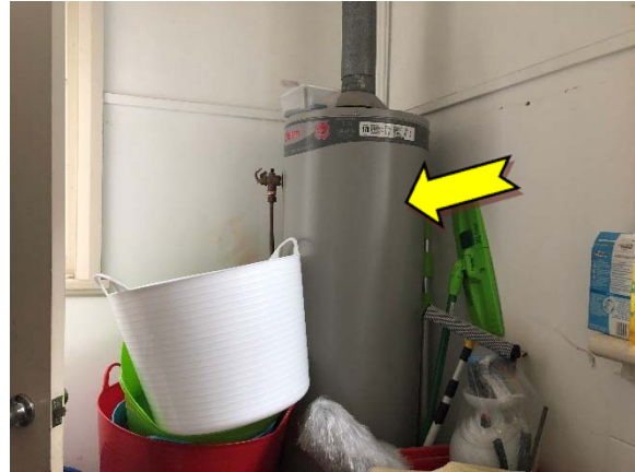
Photo 8. Interior, laundry, hot water heater – suspected SMF internal insulation material.
