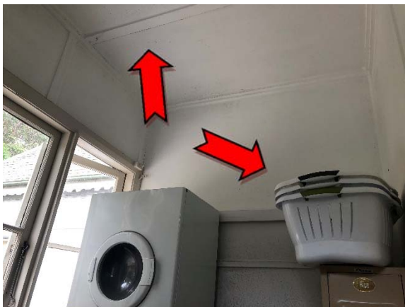
Photo 5. Interior, laundry, walls and ceiling – asbestos-containing fibre cement sheeting.
