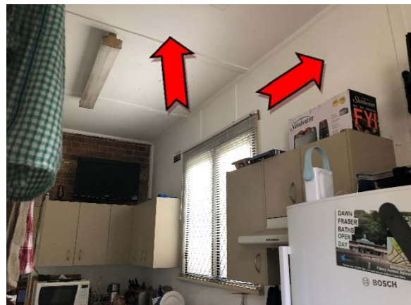
Photo 6. Interior, kitchen, walls and ceiling – assumed asbestos-containing fibre cement sheeting.
