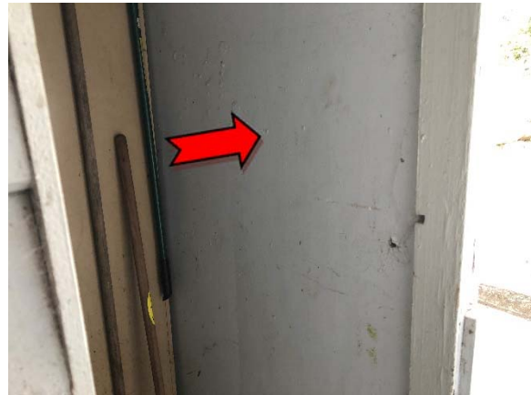
Photo 4. Interior, shed/rear toilet, walls – asbestos-containing fibre cement sheeting.
