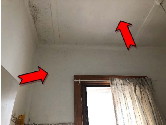
Photo 7. Interior, bathroom, walls and ceiling – assumed asbestos-containing fibre cement sheeting.
