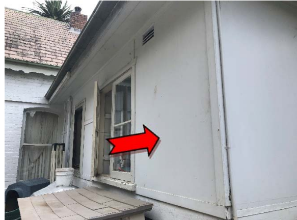
Photo 2. Exterior, rear extensions, throughout, upper walls – asbestos-containing fibre cement sheeting.
